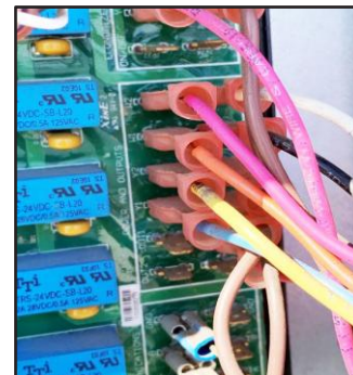
Figure 2 Surveyor Control Wire Example
